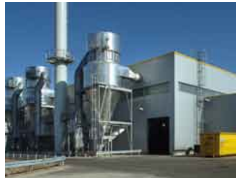
Construction and operation of Stabilat® plants
