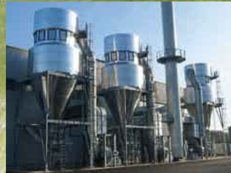
Dedusting of the machinery hall
