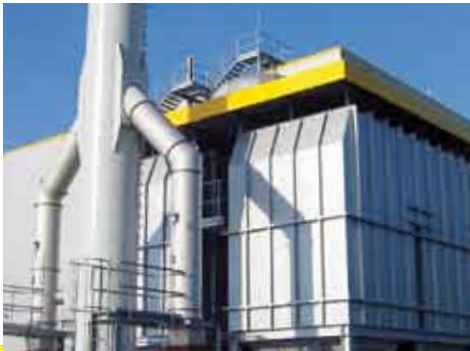
Exhaust gas purification via LARA ®
